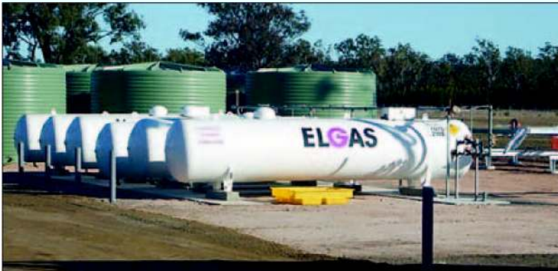
LEFT: LPG (for the steam boiler) and water storage (for steam injection) at Carbon Energy's Bloodwood Creek site, 5km from Kogan.
